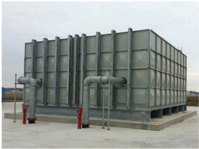
Fire reserve tank in Louisiana Airport, USA
