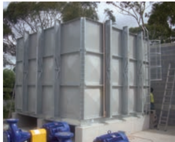
Water Storage for Cooling System at Data Center
