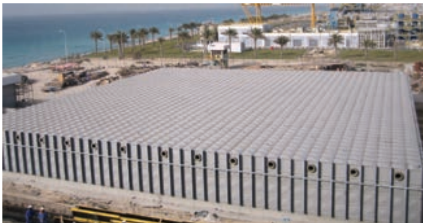
Conditioning Tank for RO Desalinated Water
