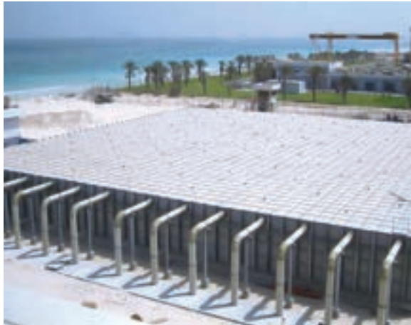
Conditioning Tank for RO Desalinated Water
