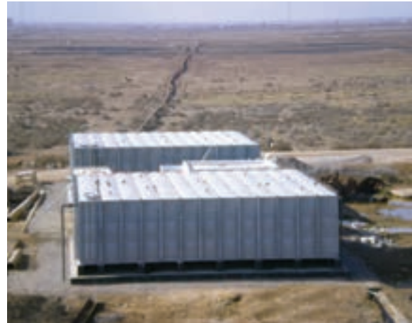
Fire Tank at Crude Oil Pumping Station
