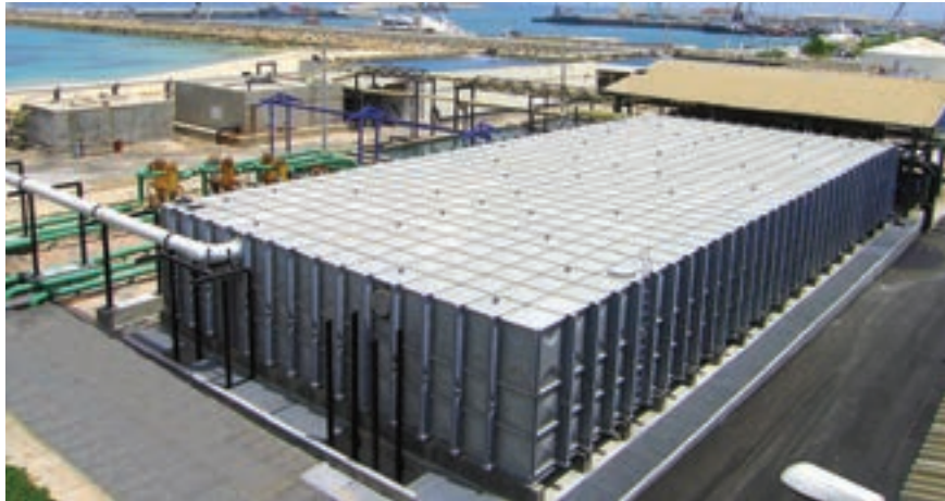
Seawater Intake Tank at Desalination Plant
