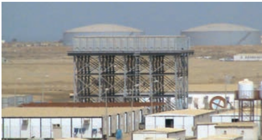
Elevated Potable Water Storage Tank
