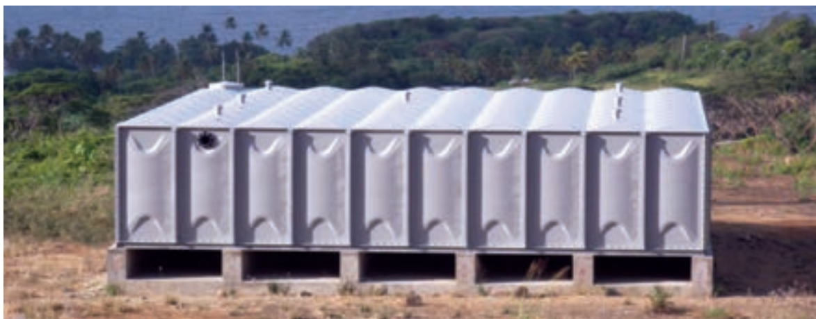
Rural Potable Water Storage Tank
