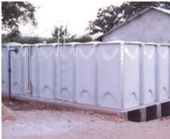
Potable Water Storage at Rural School
